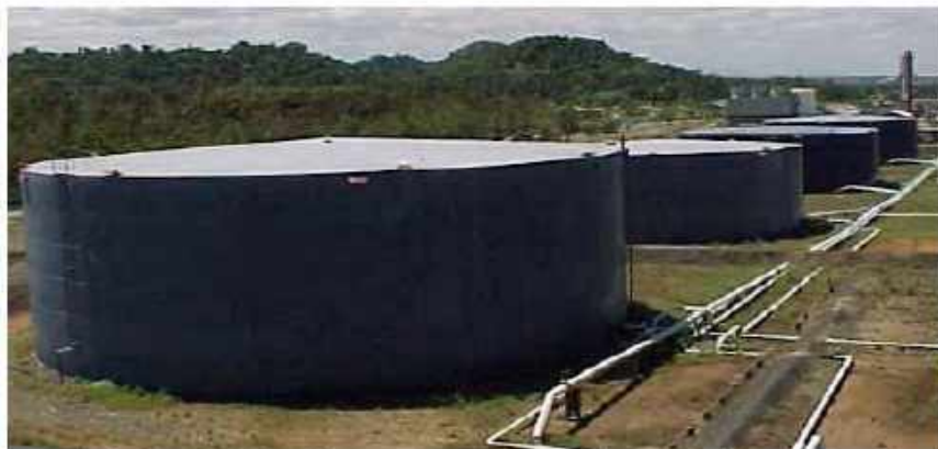
Figure 1.4. Cone roof tanks connected to pipelines (Caribbean Petroleum)
