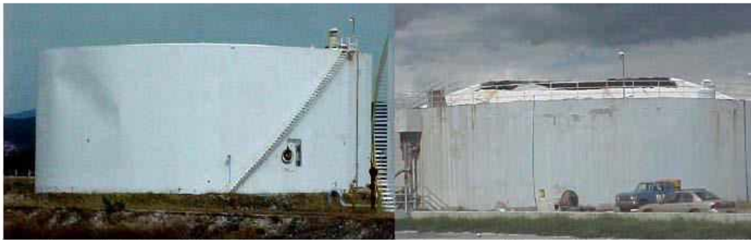
Figure 1.7. Local buckling and collapsed dome roof tank after Georges (1998), Puerto Rico.
